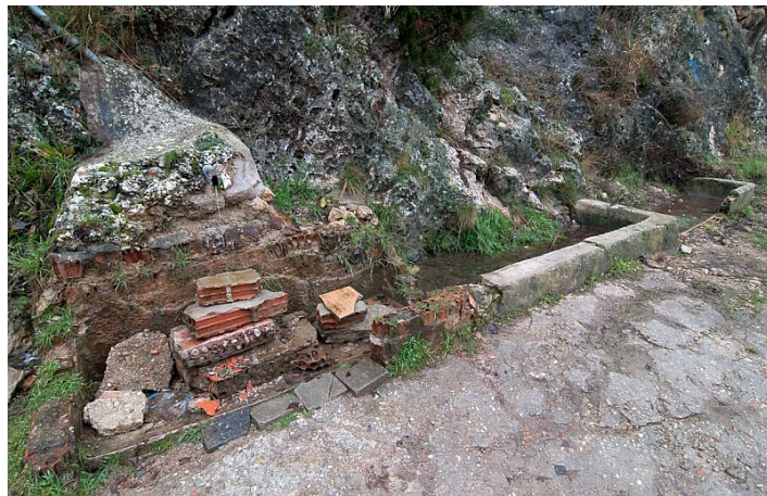
Fig. 4: Water trough before restoration. Photo: AHE.
